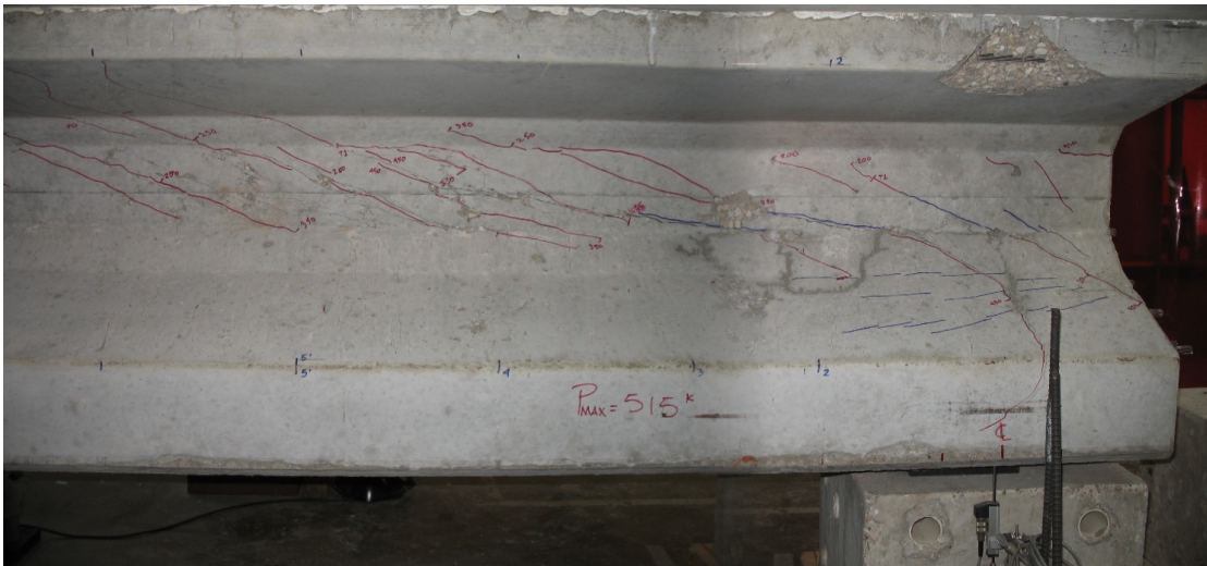
Figure 4- 29: Live end of Tx28-I at failure for Test 4.
