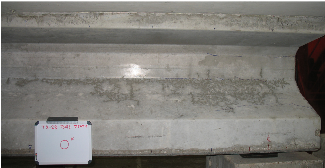
Figure 4- 18: Tx28-I dead end before Test 3.
